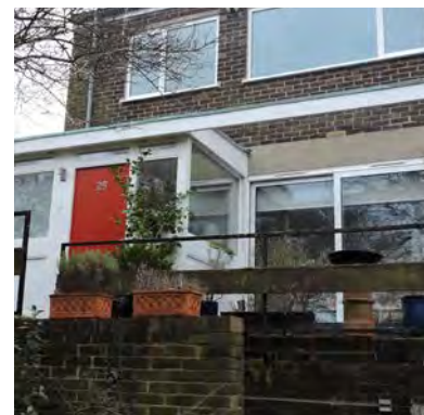
Original doors, windows and fanlights are important to local character and can be retrofitted by a skilled joiner
