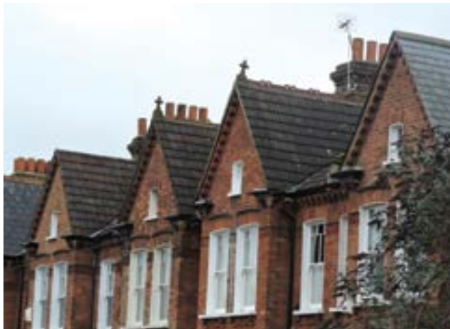
Post war concrete tiles should be replaced with original tiles
